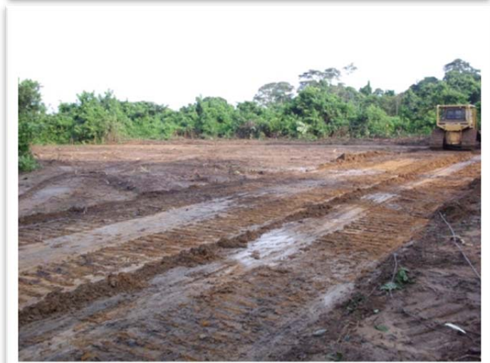
Photos from site clearing preliminary works undertaken at the location of the Lolabe Mineral Terminal in December 2013
